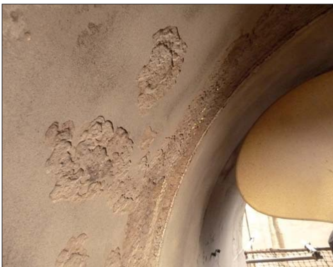
Inside of thruster tunnel with severe cavitation damage, prior to Ecoshield application.
