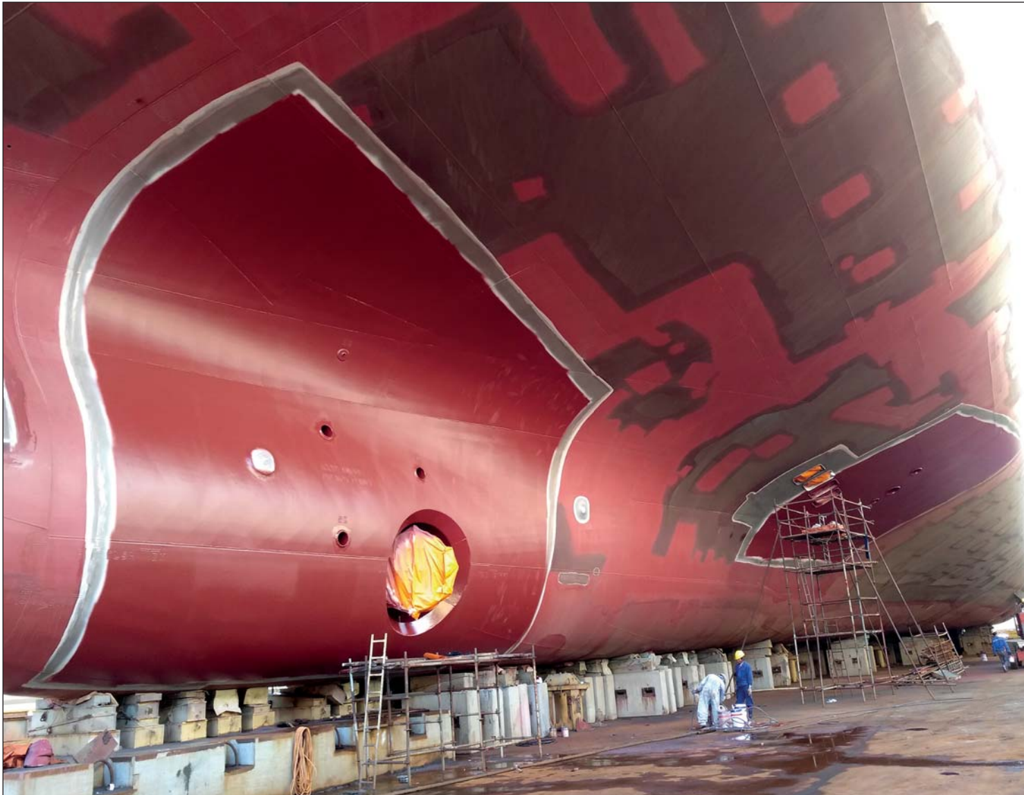
The outlets of both scrubbers of these container vessels were given the same lasting protection.
