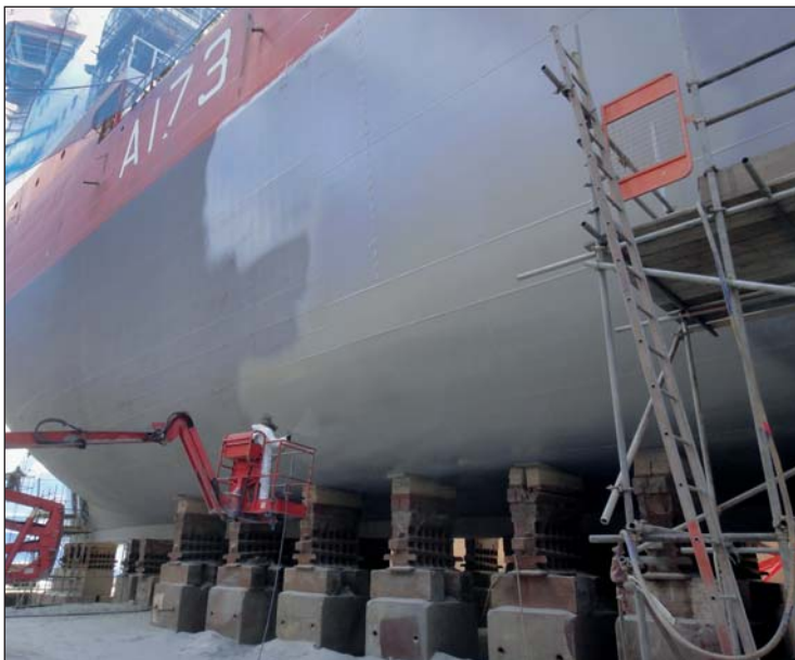
Application of first layer of Ecospeed. The coating is applied in only two layers.
