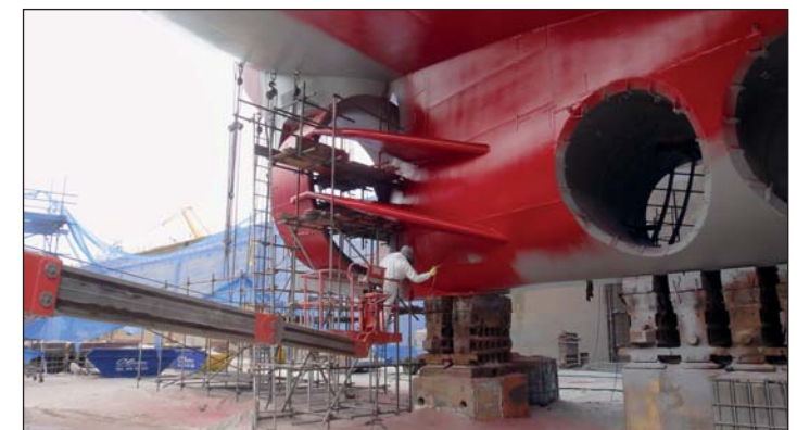
Application of second layer of Ecospeed. No repaints will be needed during future drydockings.
