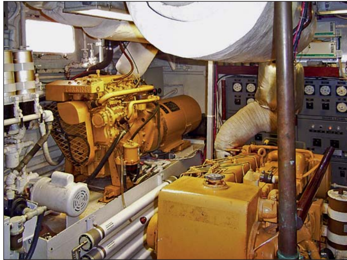
The Oceantide's engine room.
