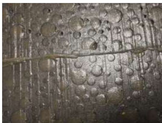
Ecofix® applied – additional application counter direction is required in order to fill all pitting
