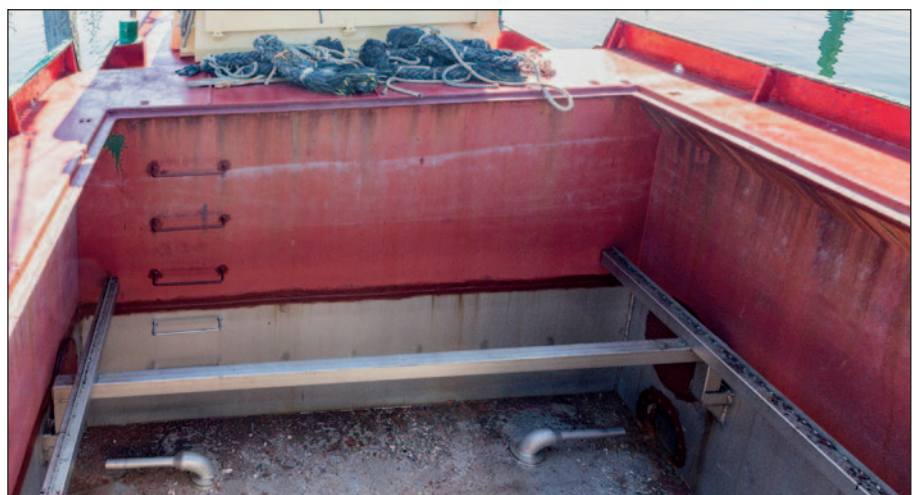
Ecospeed on the inside of the hold of the YE 48 has remained in excellent condition for over 15 years requiring only very minor touch-ups during that time.
