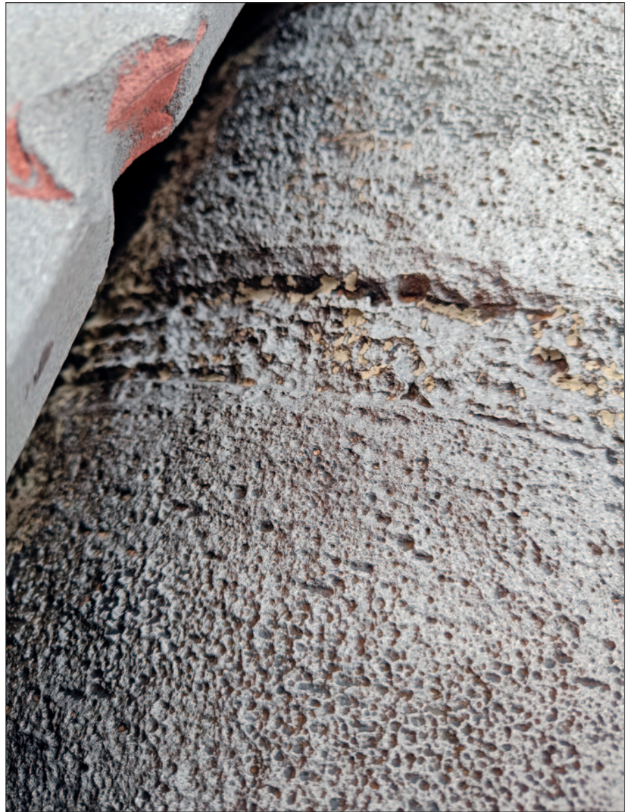
Severe pitting in rudder as a result of cavitation. Ecoshield can prevent this from happening again.
