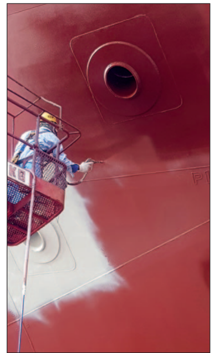
All parts of a scrubber can be given the same protection.
