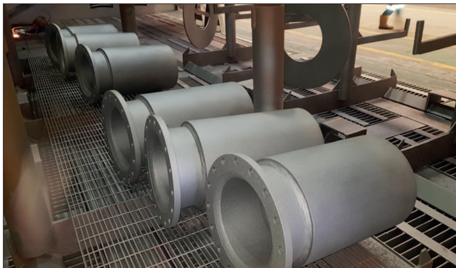
Scrubber pipes prior to Ecospeed application.
