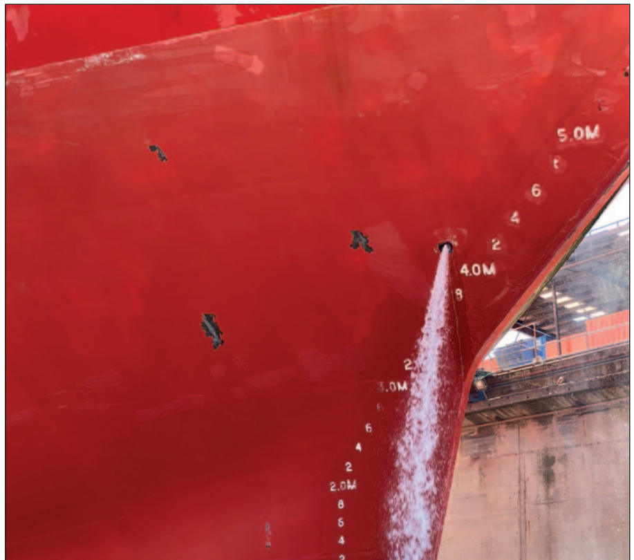
Bow area of RRS James Clark Ross after sailing in ice with Ecospeed for six years: no corrosion, only small mechanical damage from the anchor chain.
