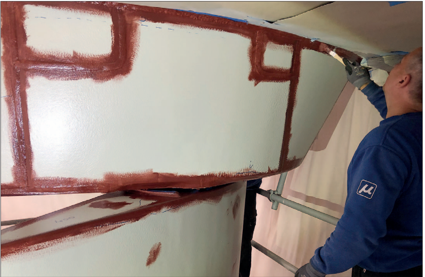
Rudder being coated with Ecoshield. The first coat (white) is complete and stripe coating is being applied prior to the final coat (red).
