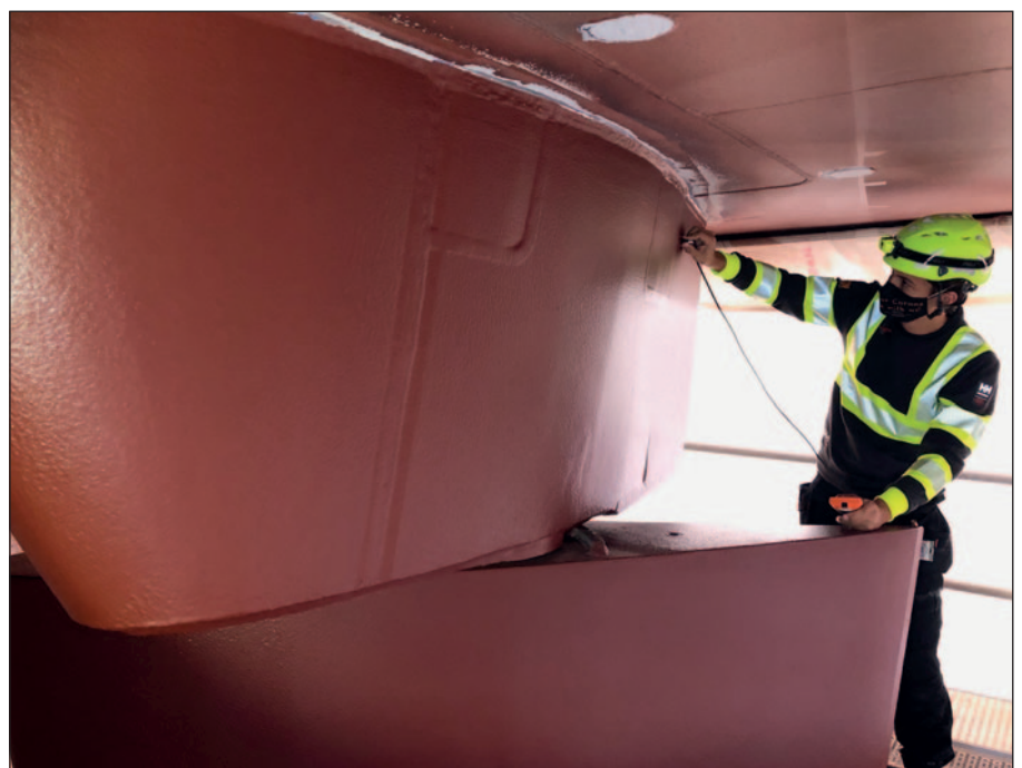
Inspector from SCICONworldwide checking that the correct final DFT of at least 1000 µm has been achieved uniformly.
