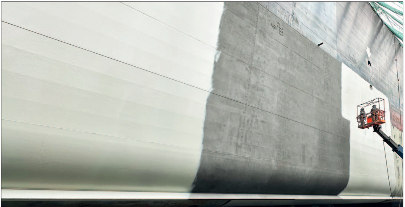
Proper preparation and application of Ecolock to FSRU conversion, essential for long-term protection of offshore assets.
