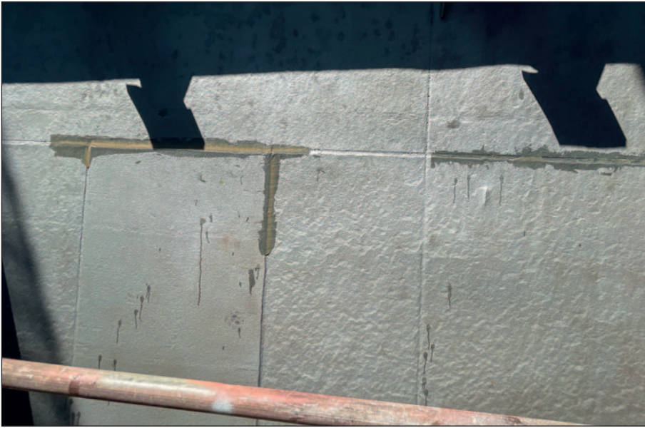
Ecofix, a filler compatible with Ecoshield, is used to repair the welds and pitting.
