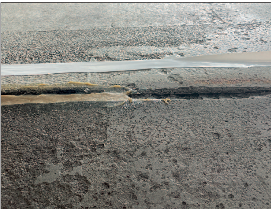
After grit blasting the inside of the hopper, the pitting and weld seams show need of repair.
