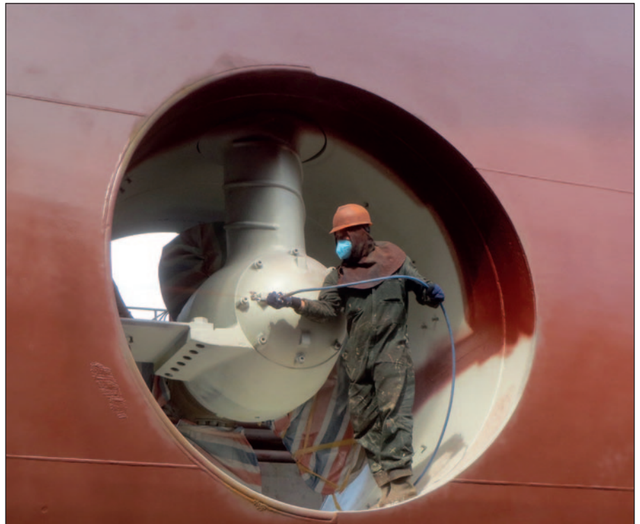
Ecoshield application on thruster tunnel. No repaint will be required during future drydockings.
