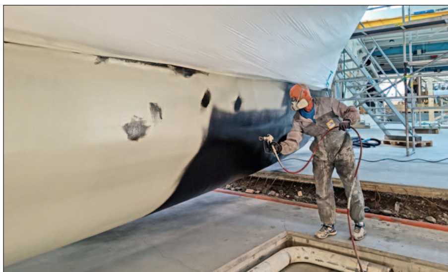
Overcoating time between layers is very short. Smaller projects like this can be completed in a single day.
