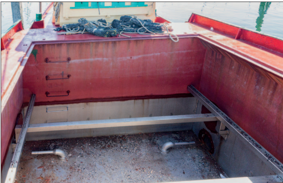
Ecospeed on the inside of the hold of the YE 48 has remained in excellent condition for over 15 years requiring only very minor touch-ups during that time.
