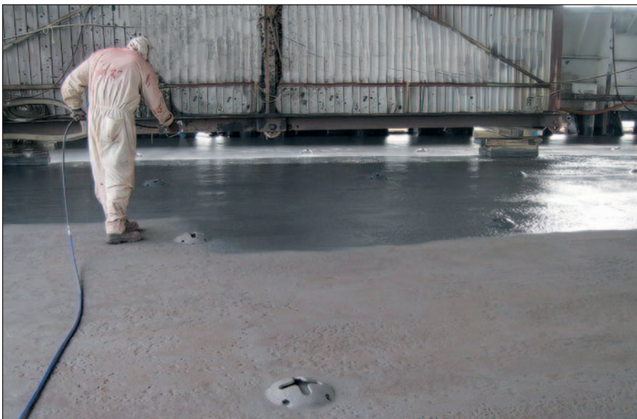
The damaged vehicle decks of the Finbo Cargo were coated with Ecospeed for protection from the heavy wear of vehicle traffic, with excellent results.
