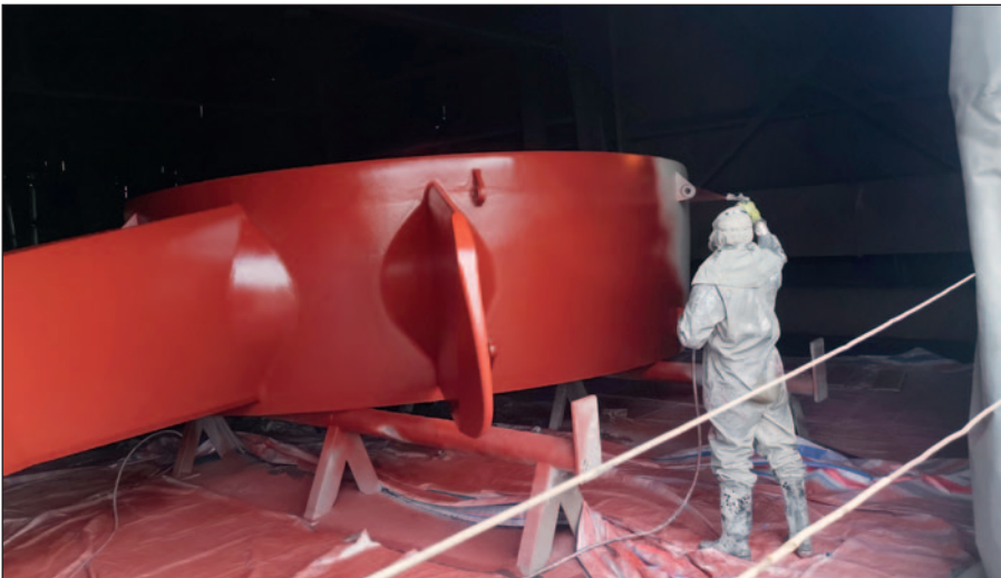
Application of Ecoshield can be done before or after installation of the running gear without any effect on the quality of the coating.
