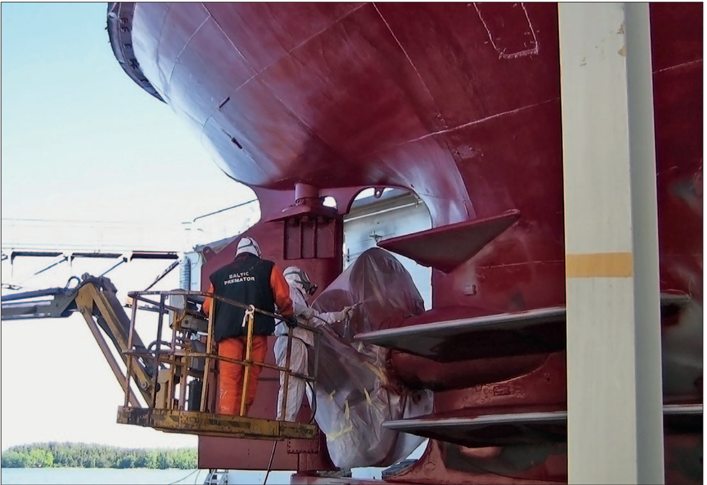
Per was the coating inspector in 2012 for the blasting and coating of icebelt and rudder of ice-breaking tug Jääsalo of the City of Kemi, at Naantali Repair Yard in Naantali.
