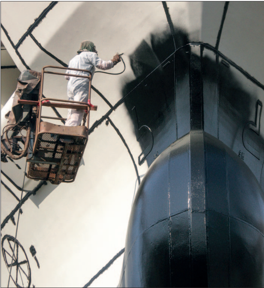
Second coat of Ecospeed being applied over a stripe coat to strengthen the protection of the welds on the Golfstrom' underwater hull.
