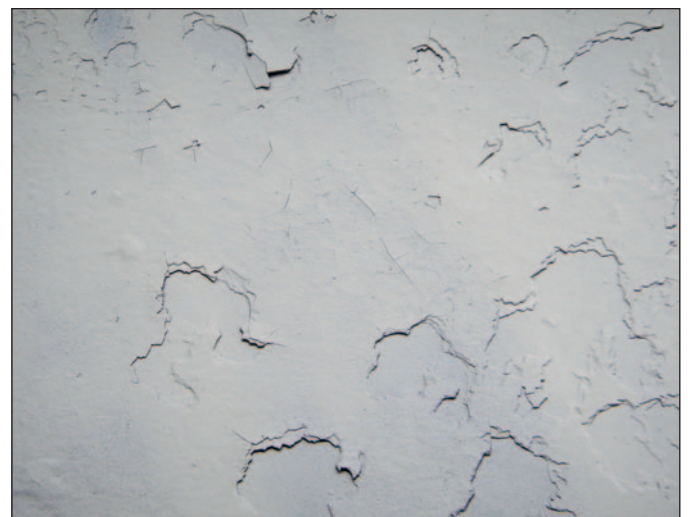
Hull of a ship where the antifouling coating has been "repaired" in drydock. This ship is about to undock.
