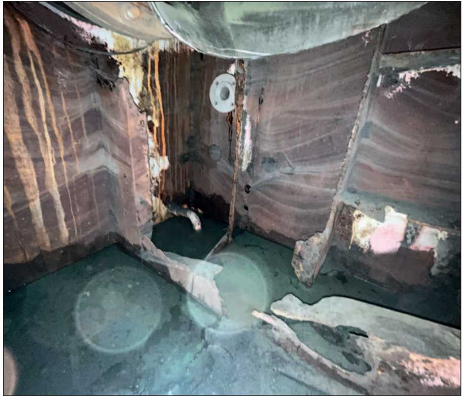
Scrubber recycle tank prior to Ecospeed application. The corrosive residue has caused severe damage to the steel.
