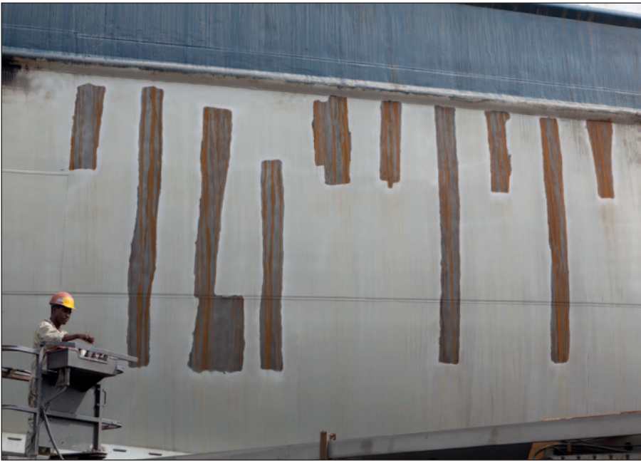
Ecospeed coated hull where hot work inside the ship has damaged the coating.
