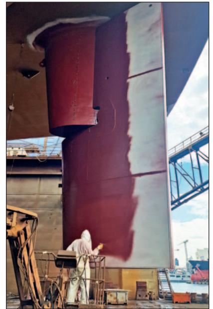
Ecoshield application is scheduled around other work on the vessel without interfering with it.
