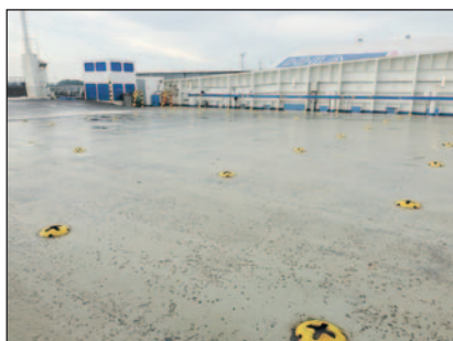
Ecospeed applied to the badly worn and pitted decks of a Ro-Ro ship. The coating was able to protect them well. The bottom photo shows the main deck after 4 years and a great deal of heavy traffic.
