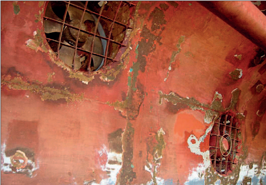
Hull of a cruise ship in drydock after 7 years with an antifouling coating.
