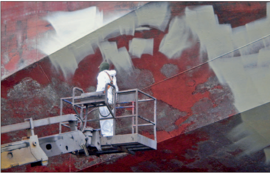
Typical repair of an antifouling coating scheme in drydock, leaving the hull rough.
