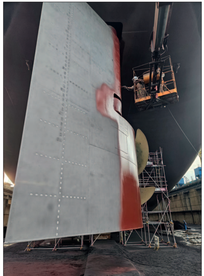
Ecoshield application is scheduled around other work on the vessel without interfering with it.
