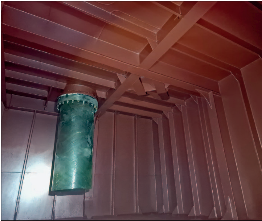
Recycle tank protected with Ecoshield.
