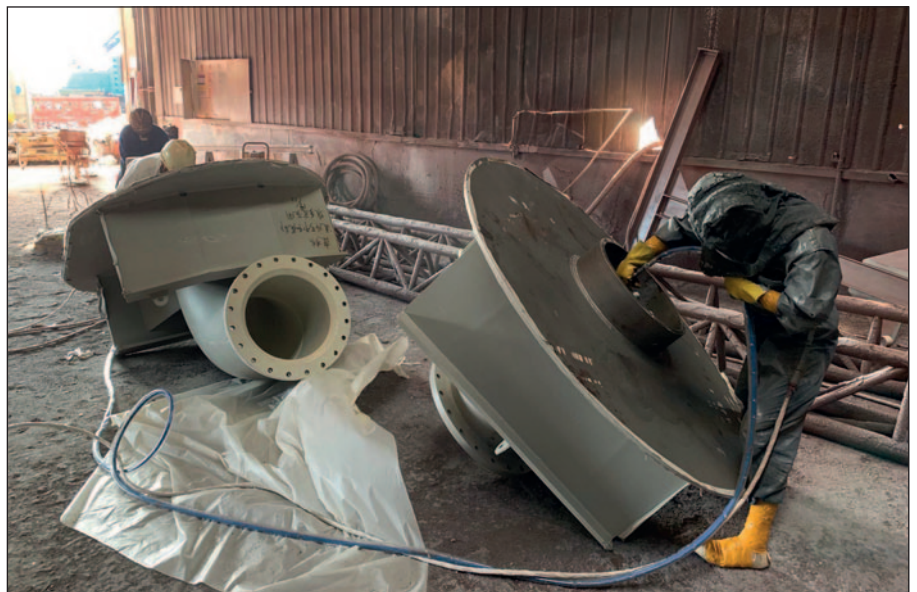
Application on scrubber system of oil tanker.
