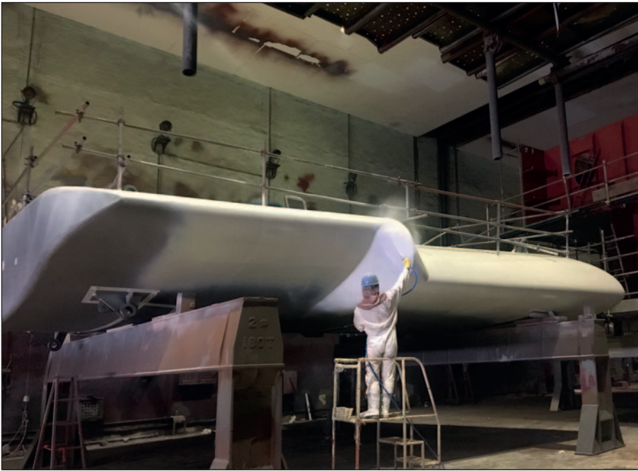
Application of first Ecoshield layer during the block phase. This has no effect on the quality of the coating.
