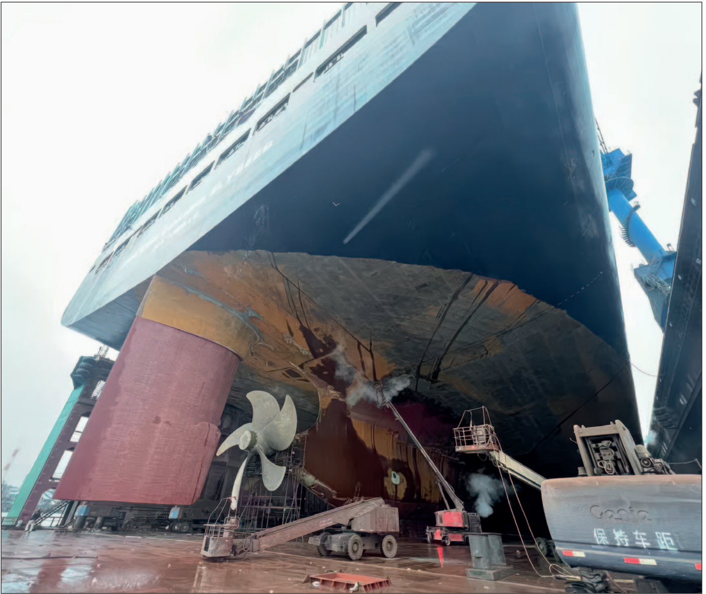
The difference between the rudder and the area not protected by our coatings is clearly visible after six years.
