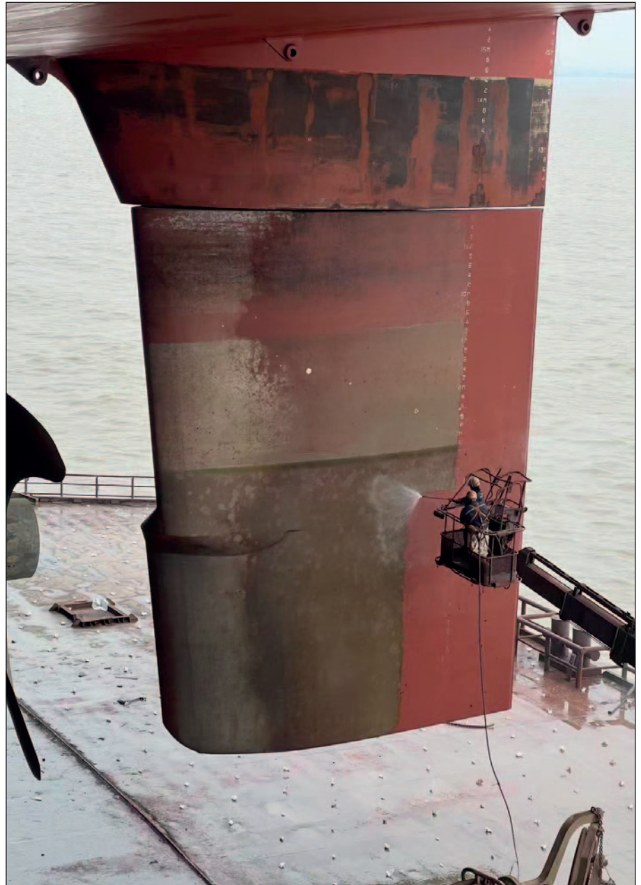
Rudder 6 year after Ecoshield application. Fouling is removed easily with high pressure washing without damaging the coating.
