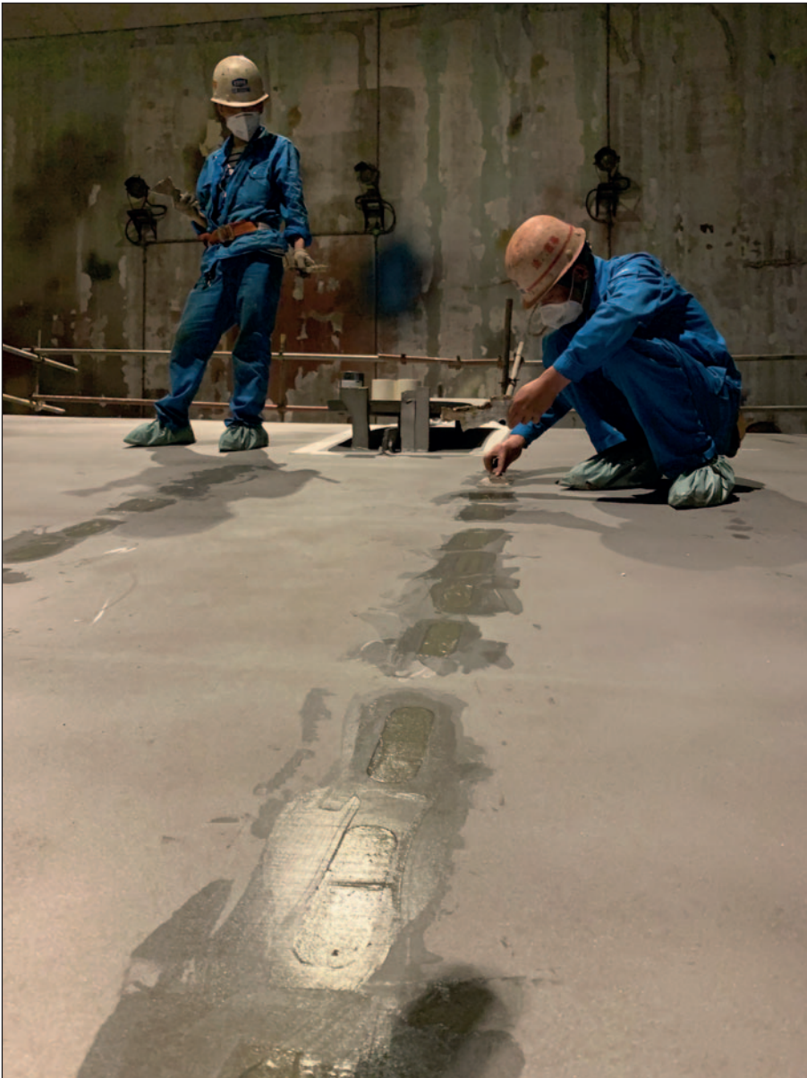
Slot welds can be filled with Ecofix, a filler fully compatible with Ecoshield.
