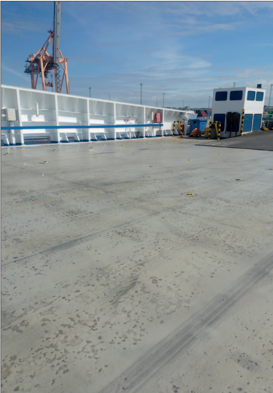
The coating on the deck is still in excellent condition seven years after application and no repaint is required.
