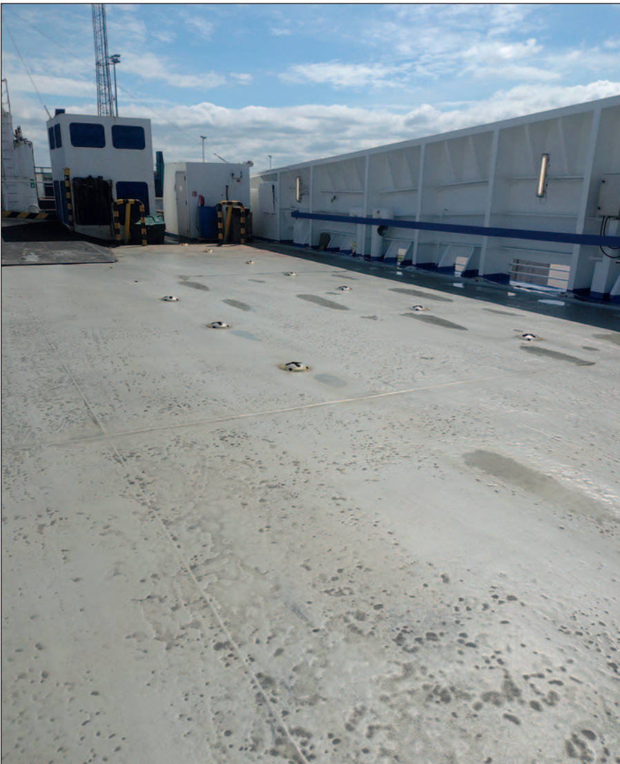
The Ecospeed coating on the deck remains in excellent condition despite continuous exposure to heavy cargo traffic and harsh Baltic weather conditions.
