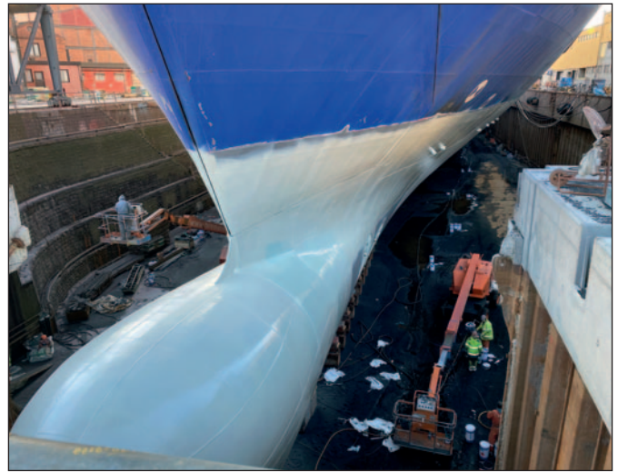
The bulbous bow and other areas prone to ice impact needed extra protection.
