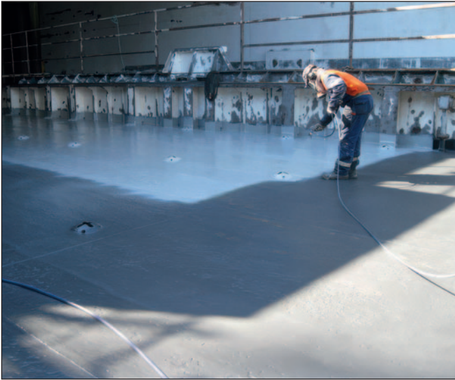
Application of Ecospeed was done in 2019 to prevent further damage from occurring.
