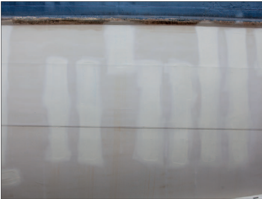
The damaged Ecospeed coated hull repaired, leaving the hull as smooth as when first painted.
