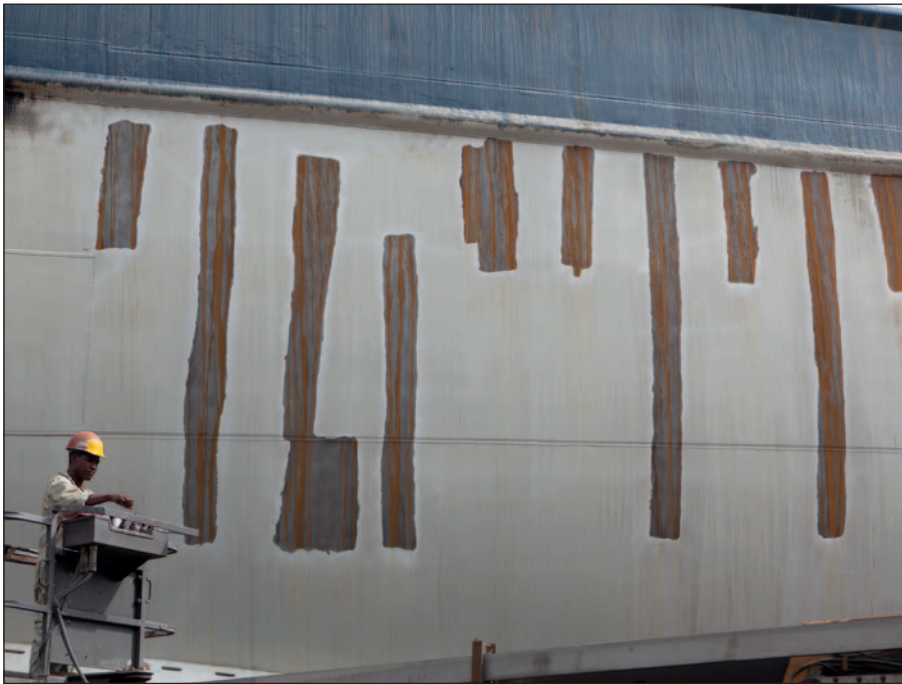
Ecospeed coated hull where hot work inside the ship has damaged the coating.
