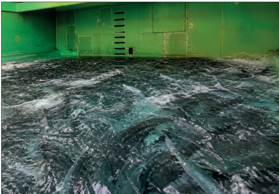
The coating on the hold of well boats is hard to maintain in the required excellent condition. Ecospeed coatings offer a solution.
